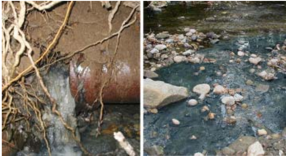
Figure 8 Raw sewage leaking from a broken pipe (left) into the Sligo Creek, which flows into the Anacostia (right). When a staff member of the Anacostia Watershed Society noticed raw sewage flowing in the creek, he notified Washington sanitation officials who claimed its source was a stormwater pipe under the jurisdiction of another agency. Continuing upstream, he found and photographed the real source of the sewage leak: a broken WSSC sewer pipe. 220 Photo source: Anacostia Watershed Society.
