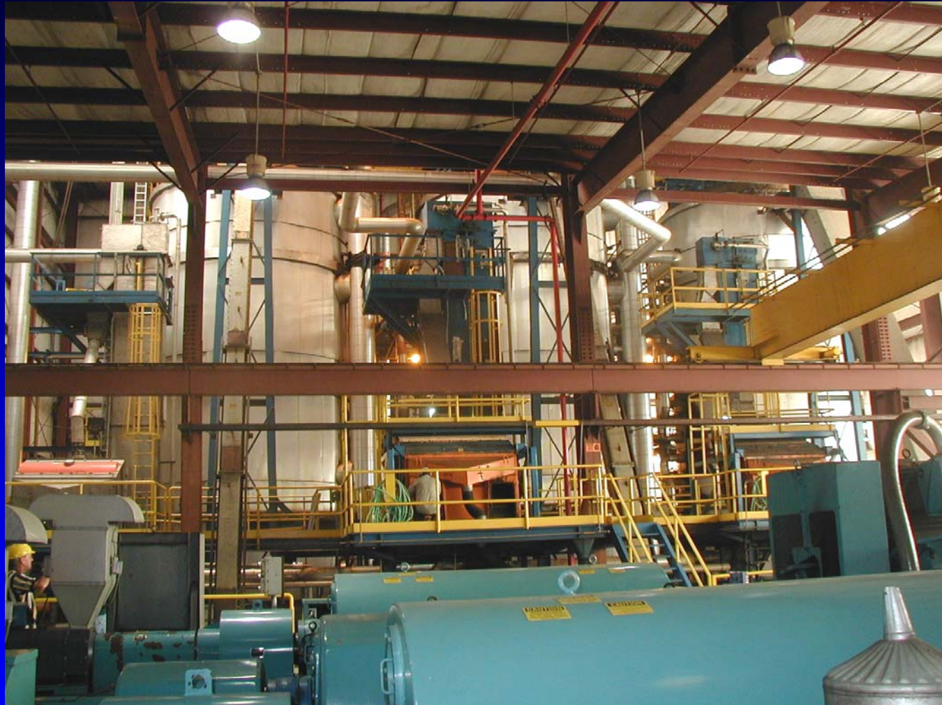
Centrifuges (foreground) and Seghers Pelletizers (background).
