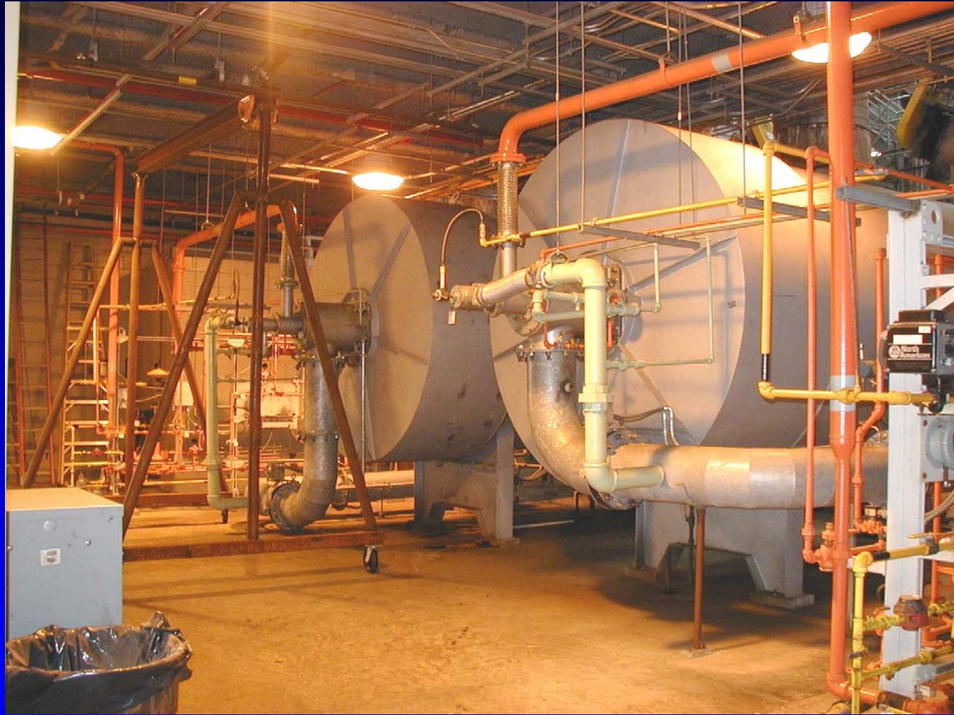
Burners (for the dryers).
