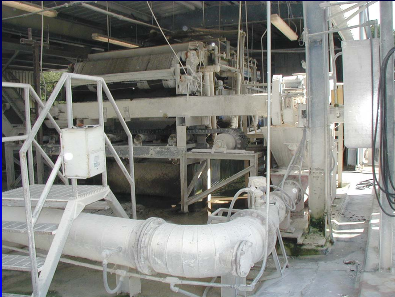
Bioset process (foreground) and belt press (background).
