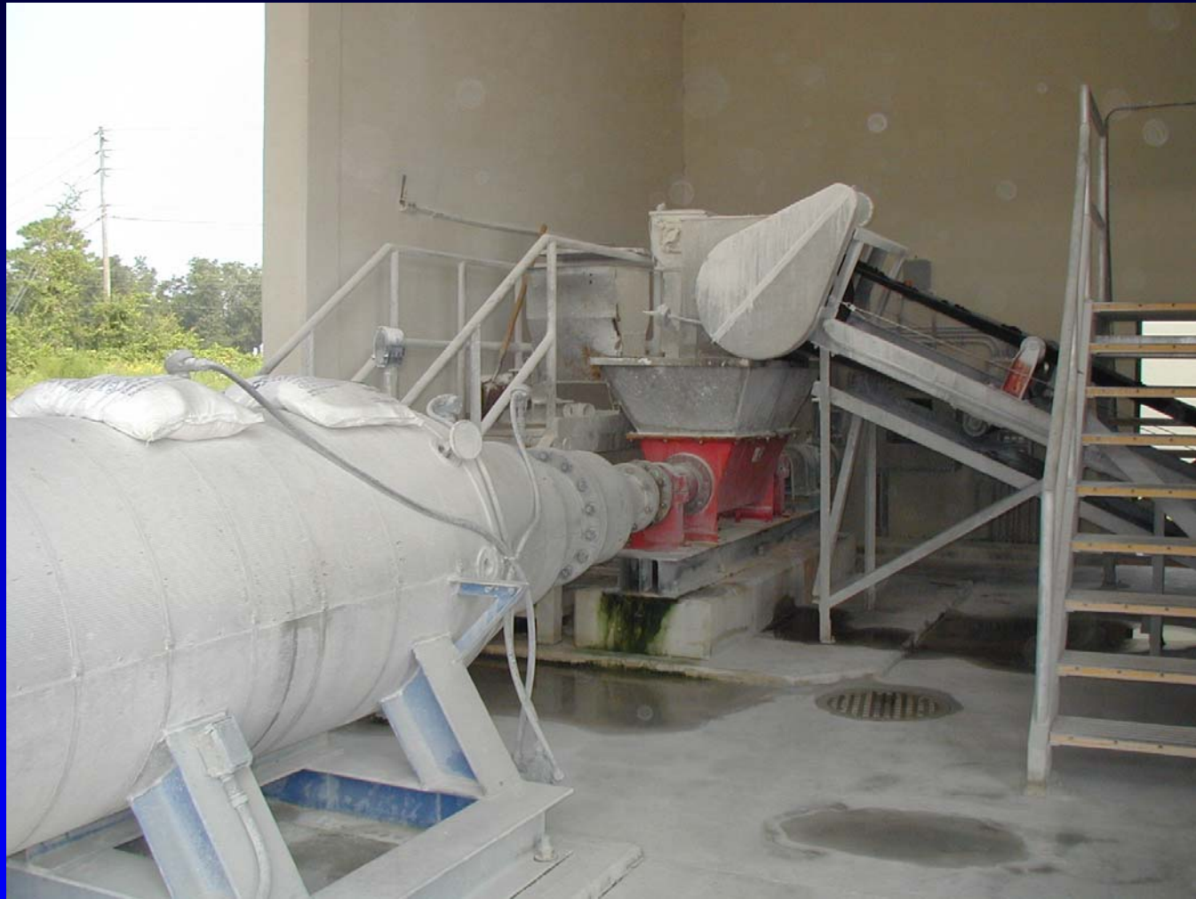
Bioset blending area (lime, sulfamic acid, and dewatered biosolids).
