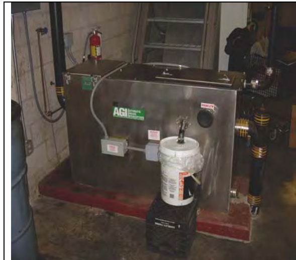
Figure 3.18 150-gpm Supplier N GRD in the RI Convention Center Basement
