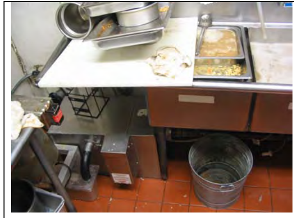
Figure 3.20 25-gpm Supplier O GRD Under a Sink in the El Tapatio Kitchen
