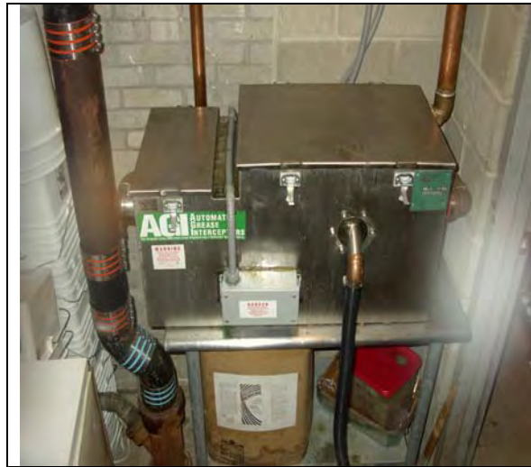
Figure 3.16 35-gpm Supplier N GRD in the L'Alouette Basement
