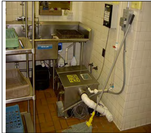
Figure 3.12 25-gpm Supplier M GRD Under the Sink in the Assisi House Kitchen
