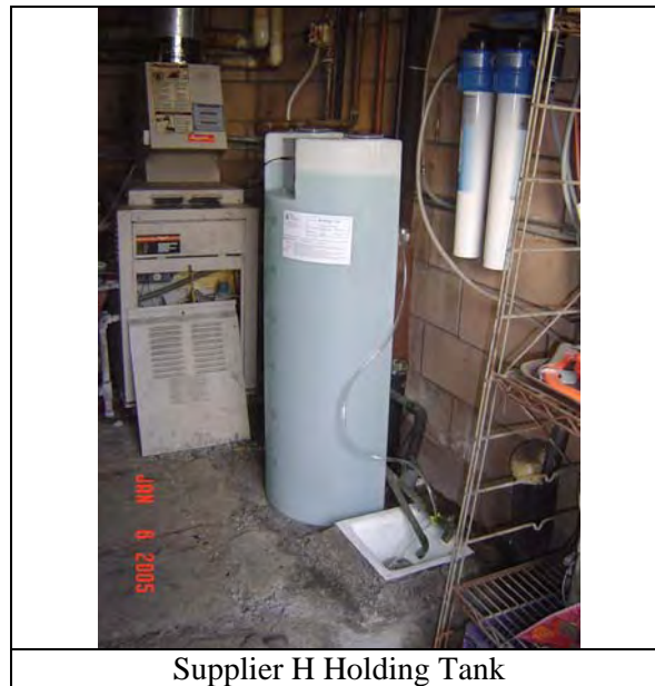
Figure 2.46 Additive Dispenser Setup at COLH HS6
