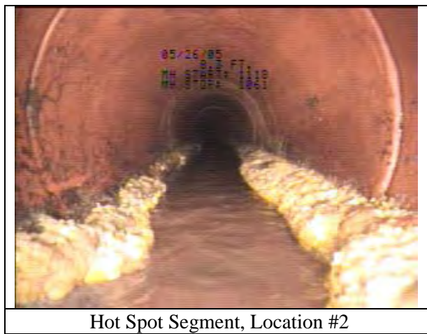
Figure 2.43 FOG Accumulation 4 Months after Cleaning
