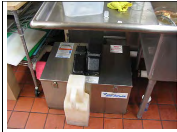
Figure 3.22 25-gpm Supplier O GRD Under a Sink in the Oh's Catering Kitchen
