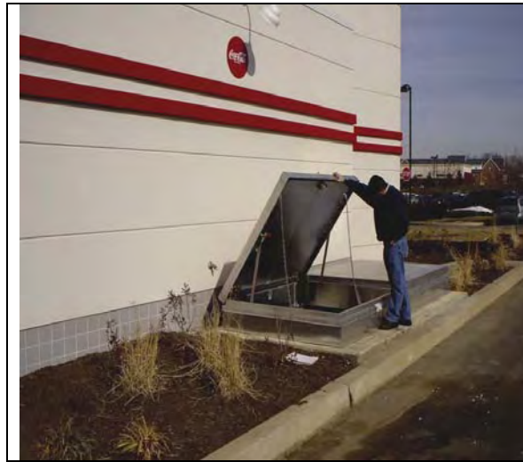
Figure 3.10 150-gpm Supplier M GRD in an Underground Vault Outside at Ruby's Diner
