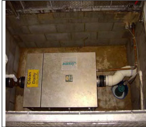
Figure 3.8 35-gpm Supplier M GRD in an Underground Vault in the Bravo Pizza Kitchen
