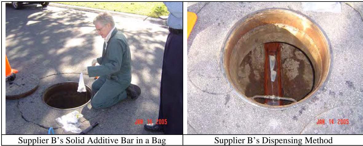
Figure 2.12 Additive Dispenser Setup at GGSD HS4
