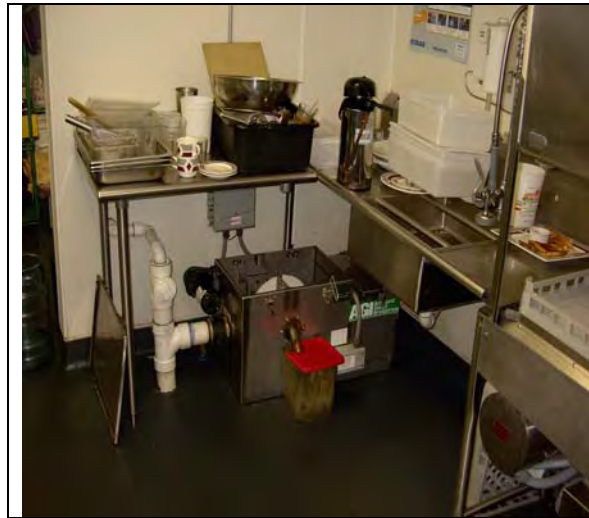
Figure 3.14 25-gpm Supplier N GRD Under a Sink in the Hi-Hat Kitchen
