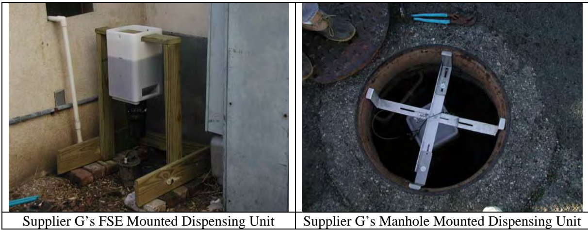
Figure 2.41 Additive Dispenser Setup at COLH HS14
