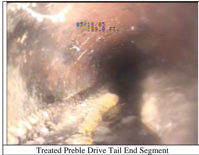
Figure 2.32 FOG Accumulation 3.5 Months after Cleaning
