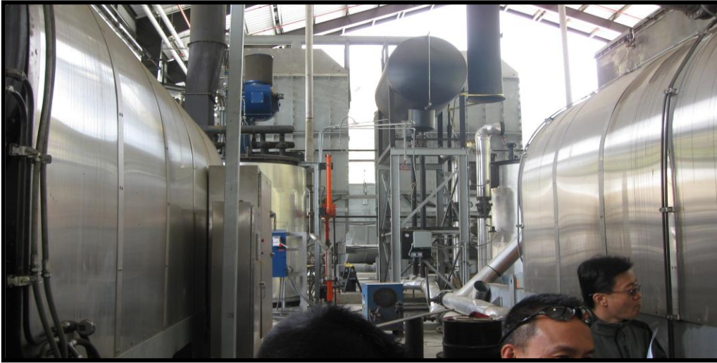
Heat Dryers at the Toland Sanitary Landfill-Ventura County
