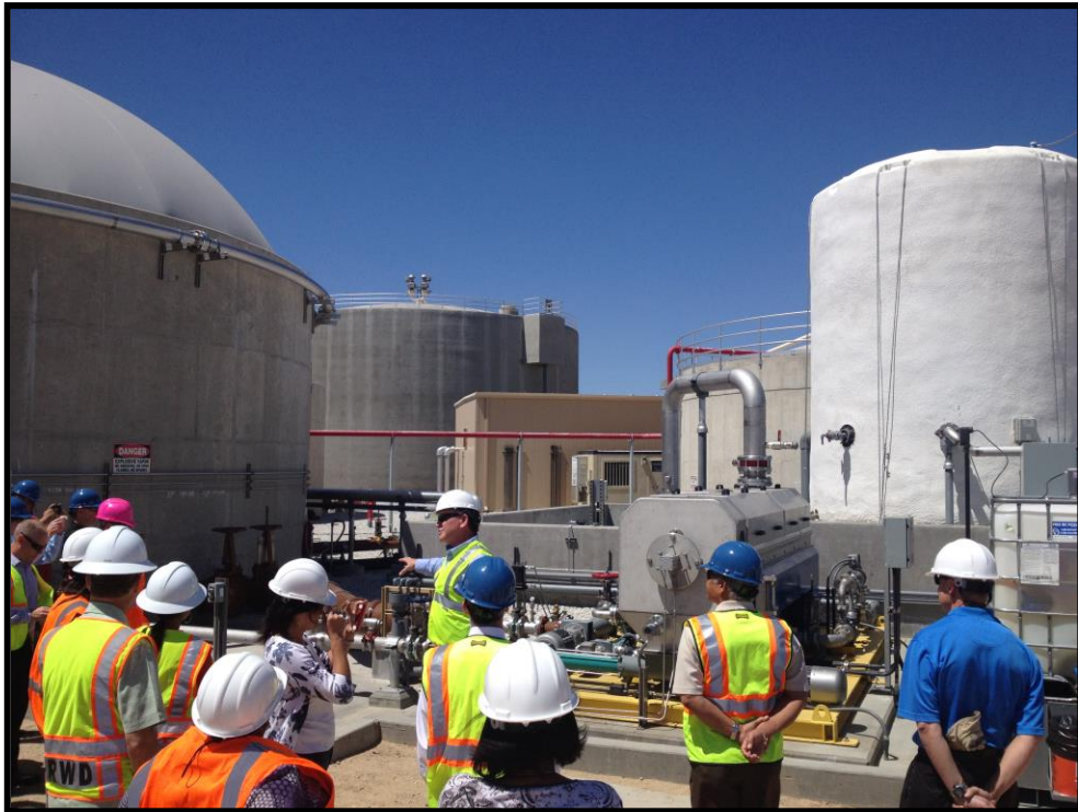
Anaerobic Digesters at Victor Valley WRA's WRP-San Bernardino County
